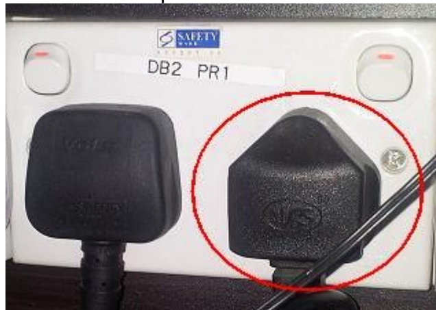
Check the power cable or sockets
